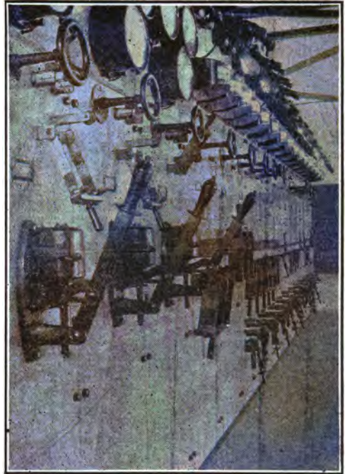
Fig. 308—The Switchboard of the New Brunswick High Power Transoceanic Station.
